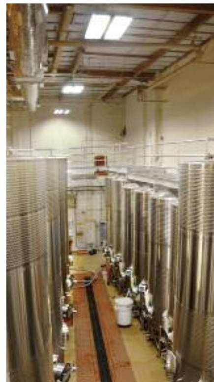
T-8 fluorescent lighting in fermentor rooms, casegoods warehouse, and barrel room reduces energy use by 58,215 kWh/year.
