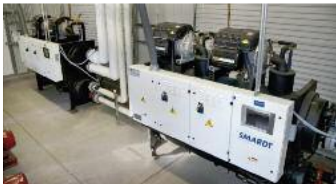
The Smardt chillers are water-cooled and have magnetic bearings, reducing friction, energy use, and maintenance costs.
