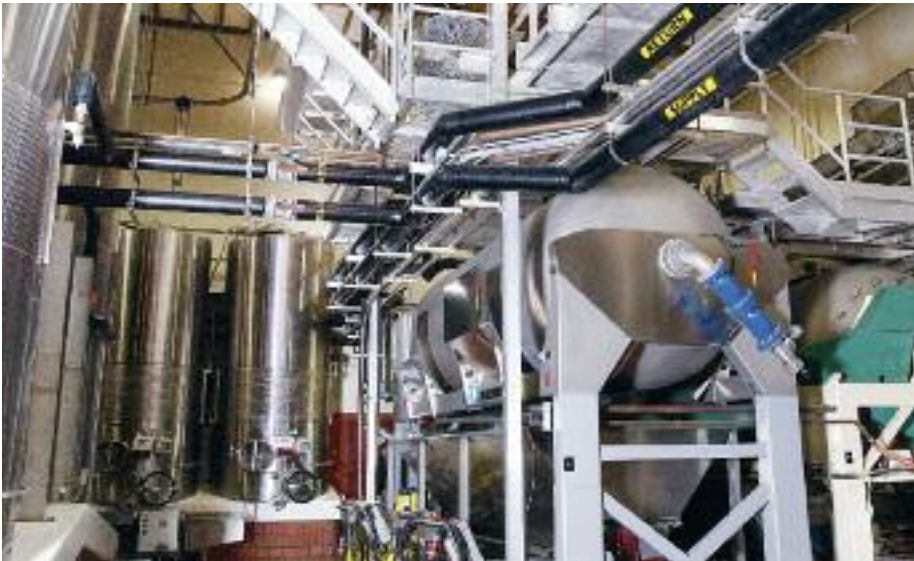
COOL-FIT ABS Plus piping supplies and returns chilled water to fermentation tanks. [Left center, above tanks] Manual COOL-FIT ABS 546 ball valves can isolate supply and return to individual tank aisles.
