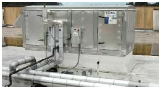
Six air-handlers atop the barrel room and five atop the casegoods warehouse, are key components of the energy-efficient new system.
